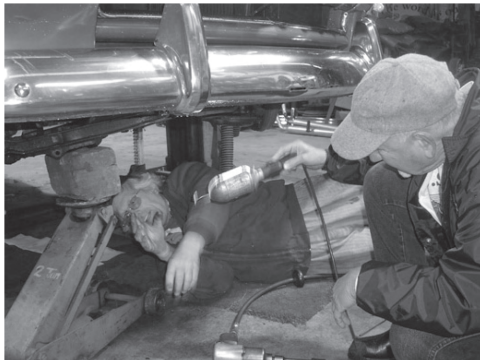
Ken VanCoelen begins the installation procedure while Dennis Fisher adjusts the light.
